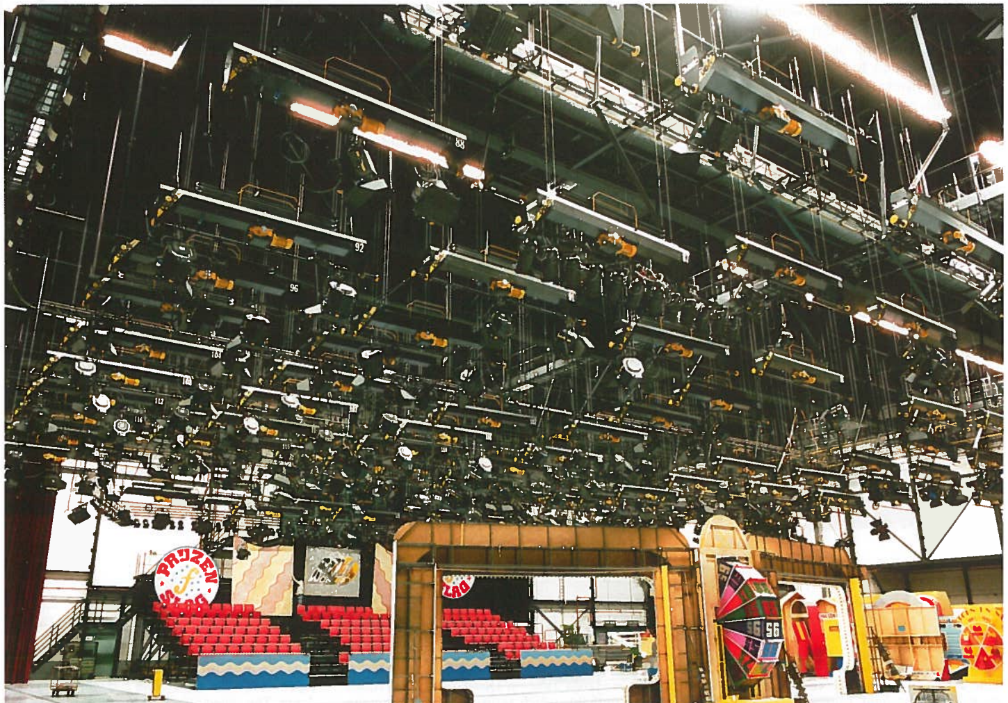
1991: Studio 22 at the NOB complex at Hilversum in The Netherlands, where DeSisti installed 136 self-climbing hoists.
