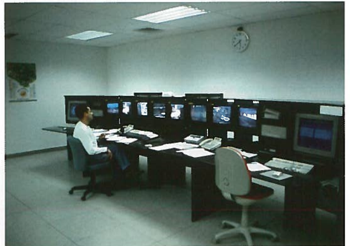
Master control room for the park-wide systems.
